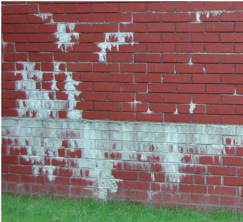
Fig. 1.10 Lime leaching on brickwork
