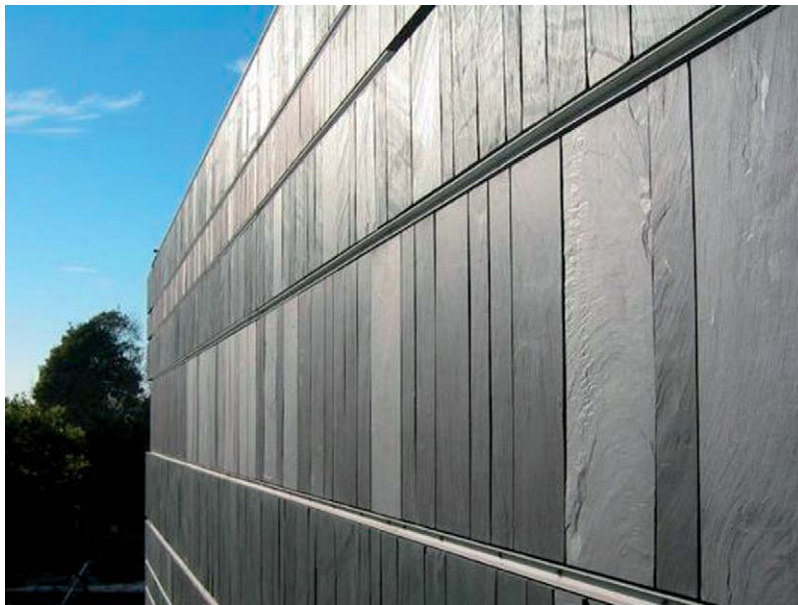
Fig. 3.18 Slate surfaced precast concrete cladding – Swansea Museum. Photograph: Courtesy of Trent Concrete Ltd
