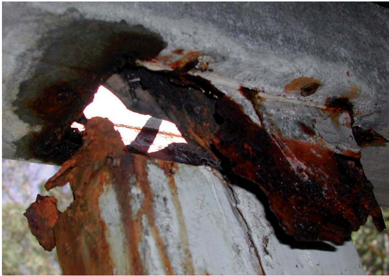
Fig. 5.35 Bimetallic corrosion between aluminium and steel
