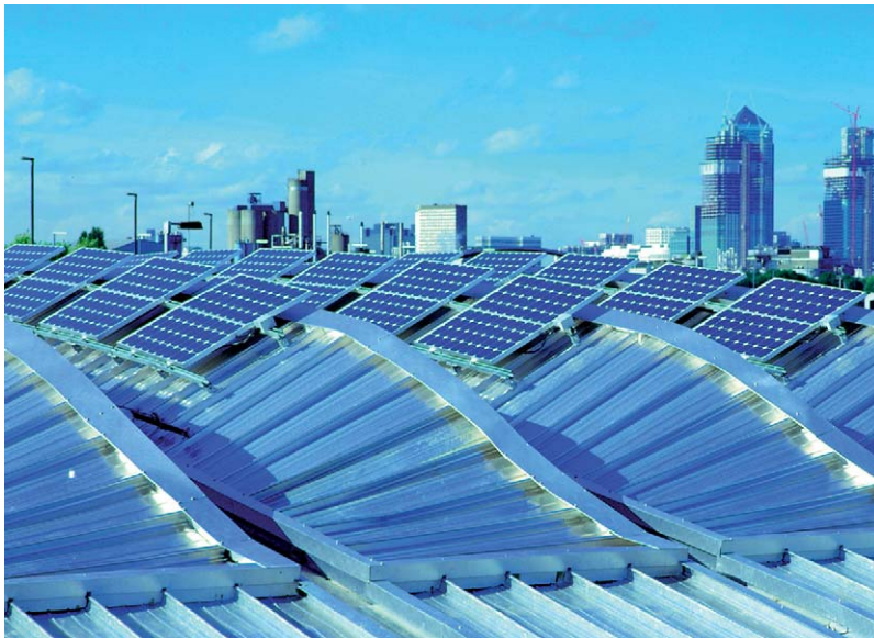
Fig. 14.2 Photovoltaic array. Photograph: solarcentury.com
