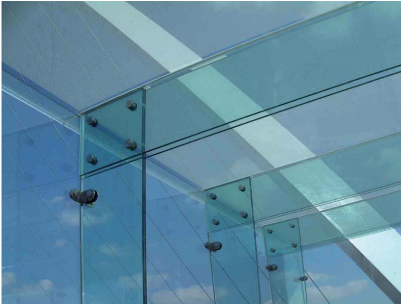
Fig. 7.22 Structural glazing detail – Gateshead Millennium Bridge Pavilions. Architects: Wilkinson Eyre Architects. Photograph: Courtesy of Wilkinson Eyre Architects
