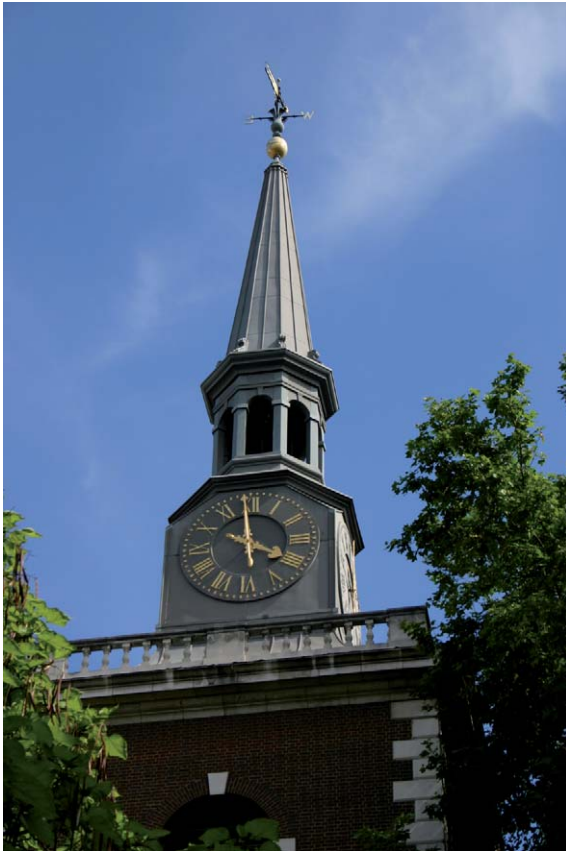
Fig. 11.2 GRP replacement spire – Church of St James, London. Photograph: Courtesy of Smith of Derby Ltd
