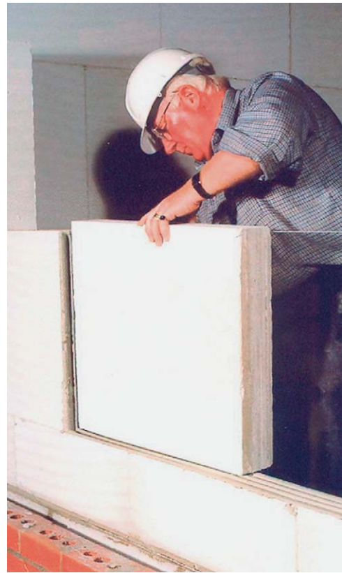
Fig. 2.3 Thin-joint masonry using large format blocks. Photograph reproduced from GBG 58 by permission of BRE and courtesy of Aircrete Products Association
