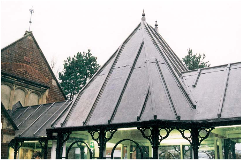
Fig. 5.25 Traditional lead roof. Contractor: Norfolk Sheet Lead. Photograph: Courtesy of Lead Contractors Association
